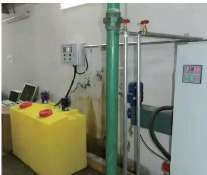
泳池药剂添加及空调制冷 Pool Sterilization
